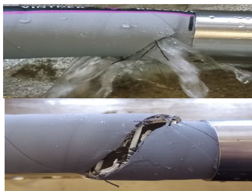
Hose burst and burst area close up
