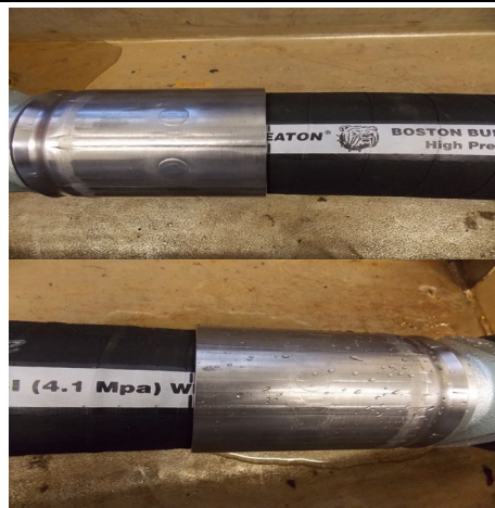
E1 and E2 prior to heat soak and pressurization
