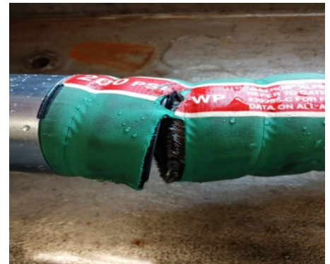
Hose burst near E1
