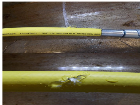
Hose burst and burst close up
